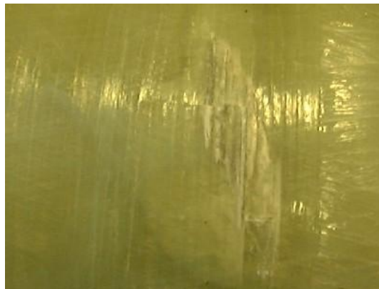
Figure 3a — Impact damage in combination with delamination and surface defects – not acceptable
