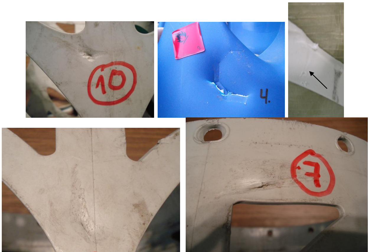
Figure 3c — Damage on casing cylindrical area – not acceptable
