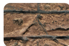
Fire Cracked Red Liner
